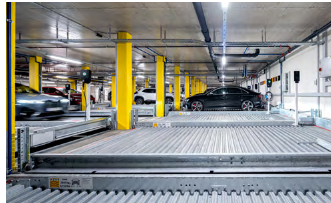
Thanks to the underground parking system from WÖHR, more space is freed up above ground for pedestrian walkways and recreational areas.
