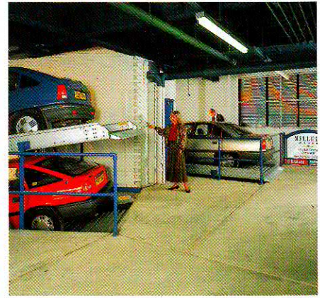
Wöhr Parklift 402 in "Miller's Wharf"
